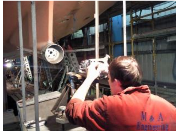
Optical alignment of the shaft path prior to line boring and installation of new cutlass bearings
