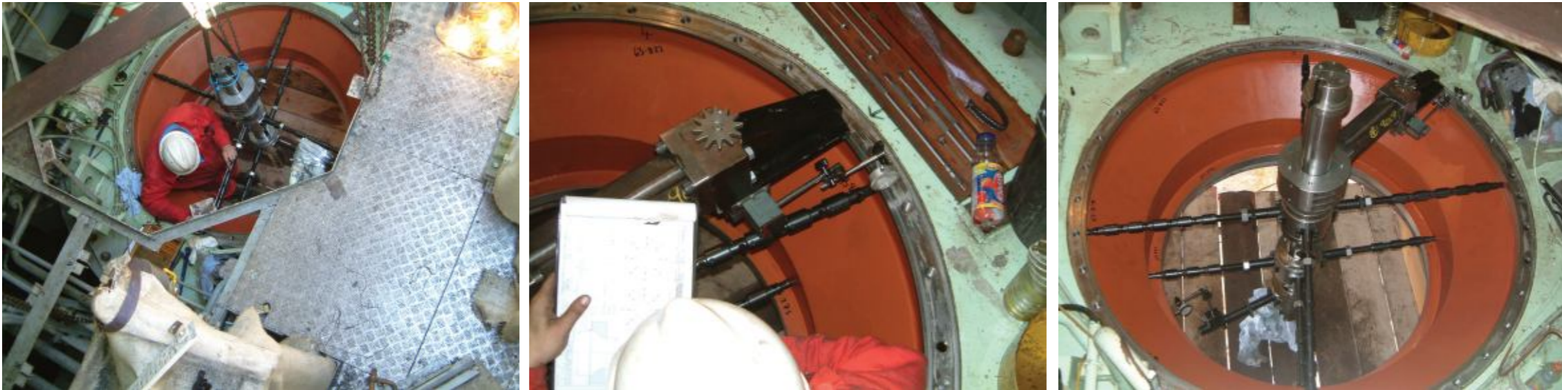
Dimensional survey, prior to re-machining a propulsion unit location using M & A's unique modular boring system.
