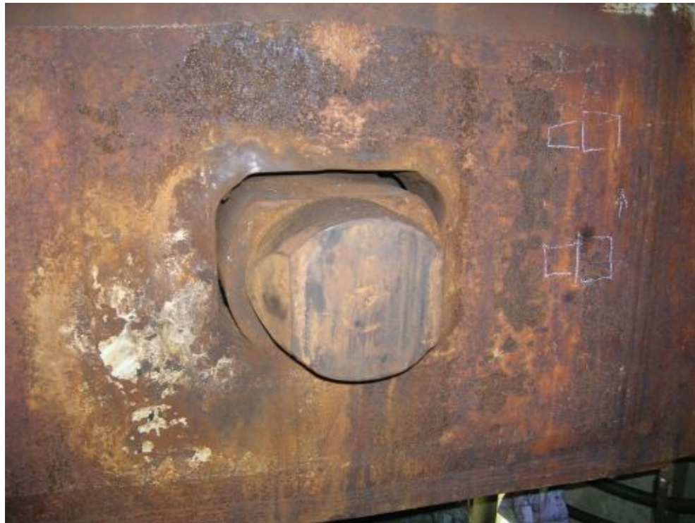
Worn pin and location
